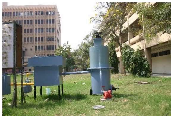
Figure 2. Gasifier and sand filter
